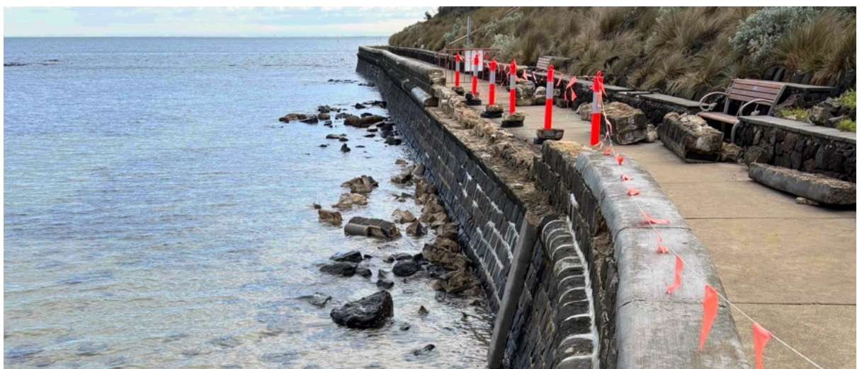
Figure 11. The same section of the coastal promenade that is shown in Figure 10 – after repairs. Maintenance can be expected to be ongoing. Photographed following a further storm on 6 th June 2026.
